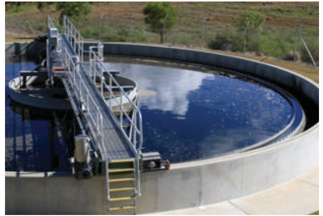
Wastewater treatment plants: one of the typical applications for the CBHSP
